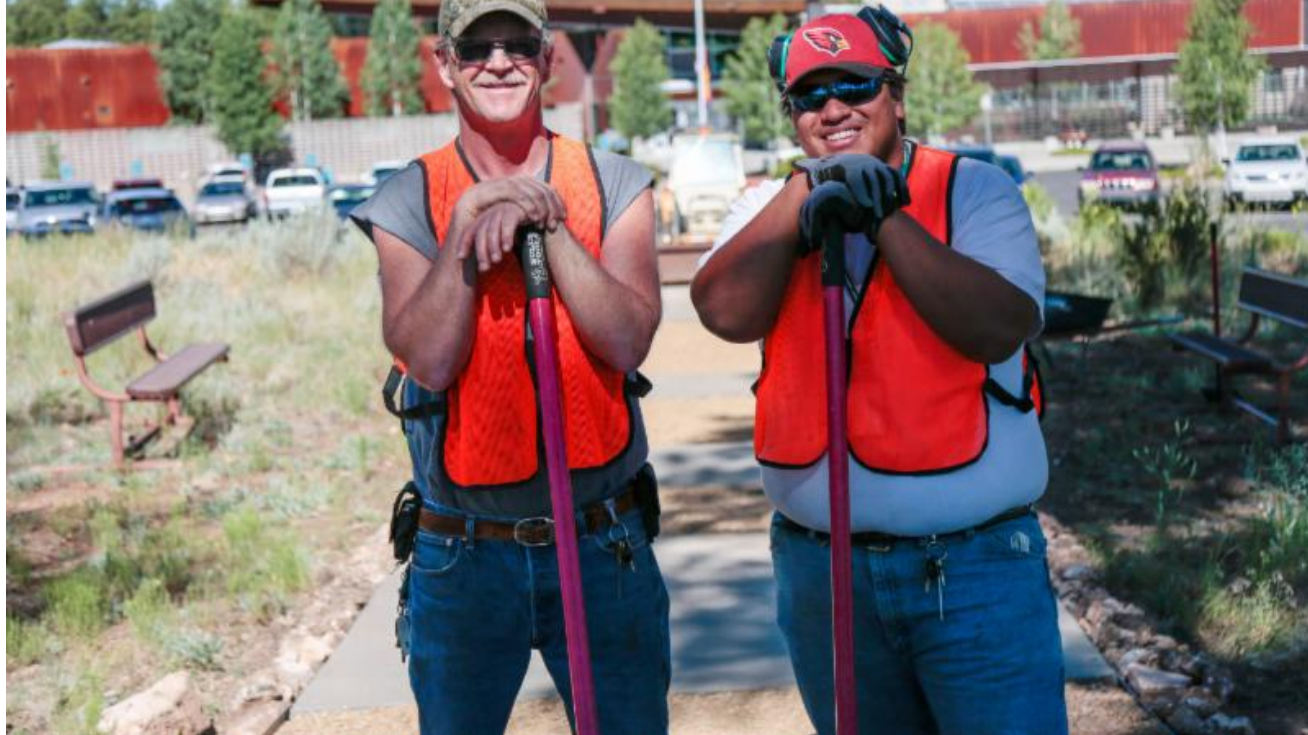
Wesley Scott and Andrew Ohumukini stand in front of the walkway project that they have been working on for two weeks.
